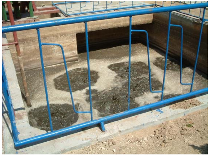
Rizhao. Liquor Factory of YAO WANG GROUP, Waste Water Treatment System
